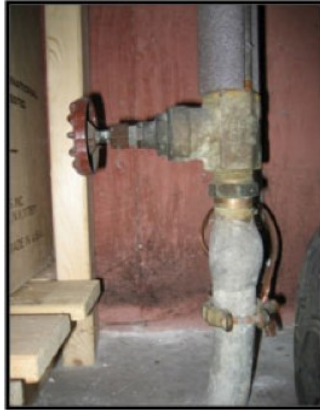
Bulb shaped connection on a lead service line. (photo courtesy of US EPA Region 5)
